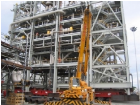
Figure 1 Fully fitted-out PAM
